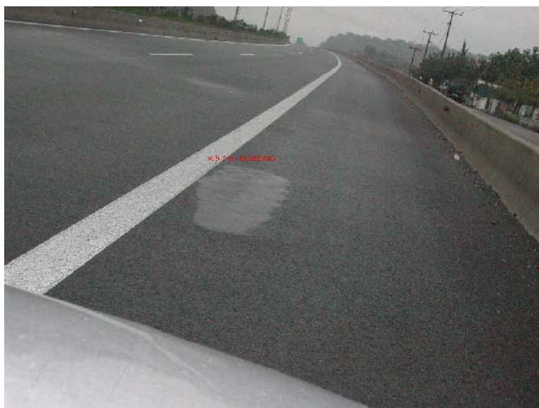
Photo 3 RC Ch.241 (Bleeding)
