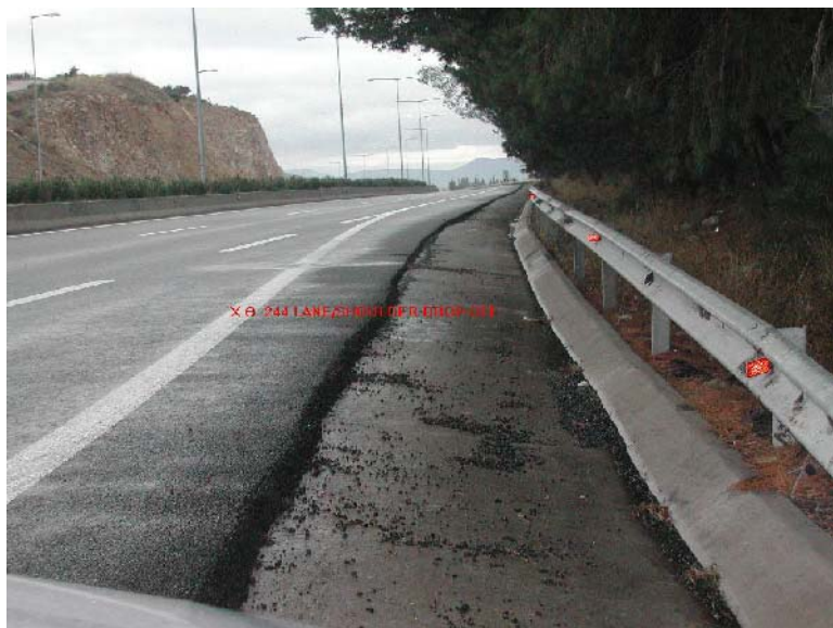
Photo 2 RC Ch.241 (Lane/Shoulder Drop-Off)
